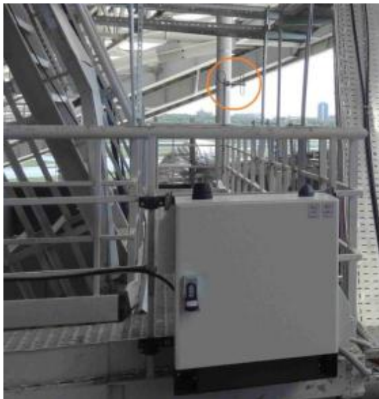
Figure 13. OMS located in Kazan Arena stadium (orange circle shows antenna of MOTOTRBO emergency channel system)
