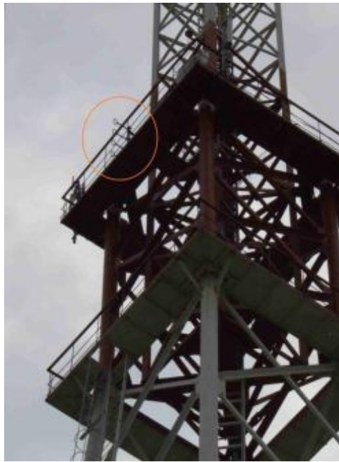
Figure 5. Antennas of service radio communications repeater on a telecommunications tower
