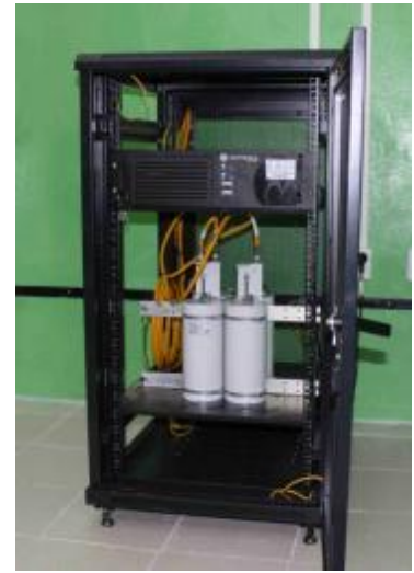
Figure 6. Equipment of service radio communications repeater
