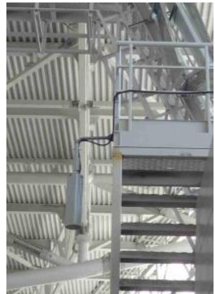
Figure 14. OMS antenna located inside Kazan Arena stadium
