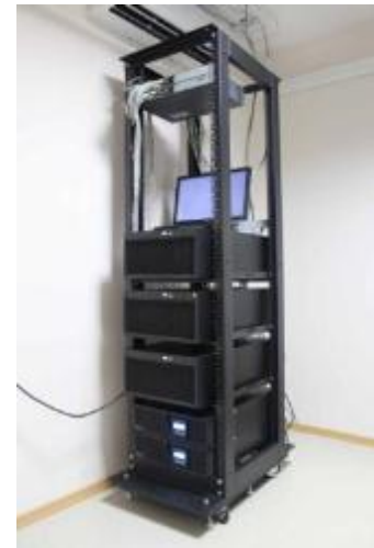
Figure 4. Server equipment of the system control center
