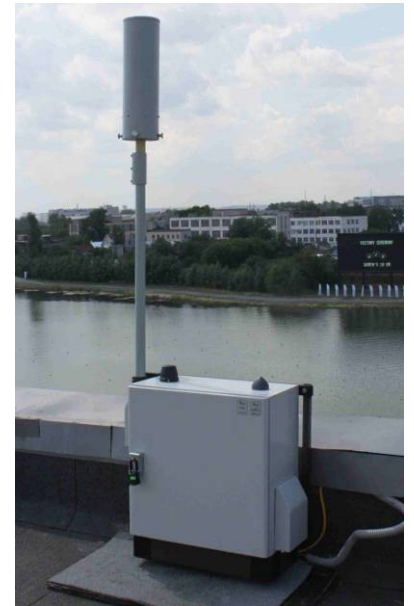
Figure 12. OMS located on the roof of Rowing Sports Center
